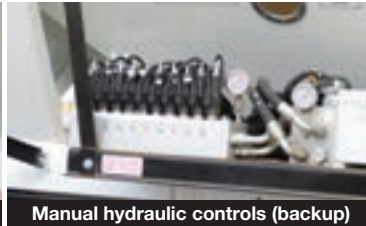
Manual hydraulic controls (backup)
